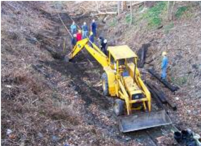
Catskill Mountain volunteers use a backhoe to replace ties during the Kingston trackage restoration in December 2006. Ernie Hunt
